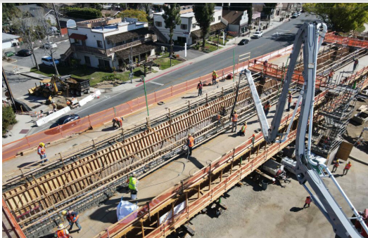
Crews completing the seven-hour concrete pour for the internal walls of the super-structure at Bonita Ave./ Cataract Ave.
